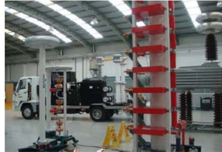
VLF-200 HVCD mobile system during the conformance testing
